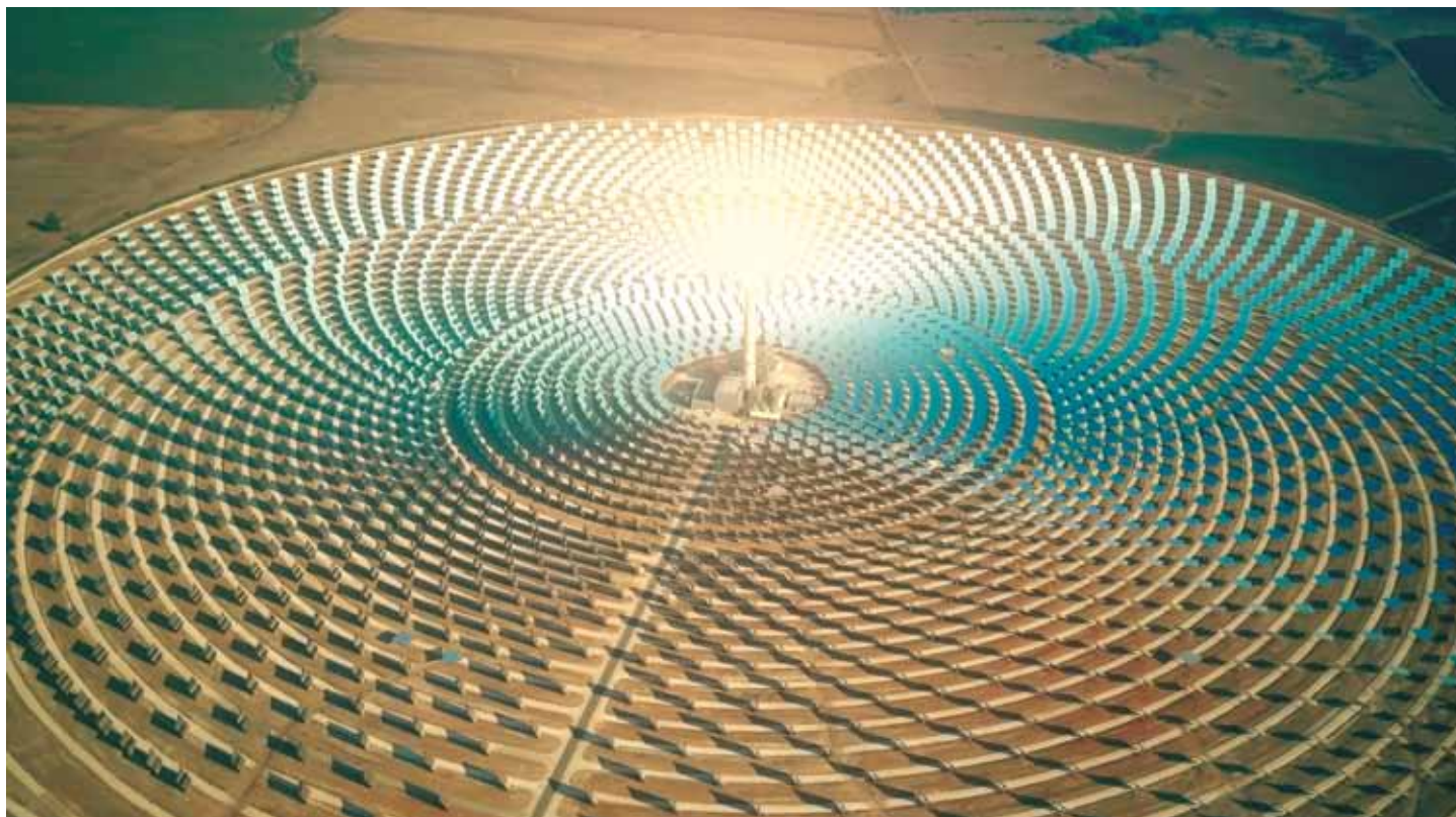
Gemasolar concentrated solar power plant in Fuentes de Andalucía, Spain, utilises a molten salt heat storage system.
