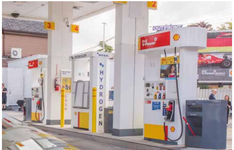
Hydrogen fuelling station. Photo: Shell
